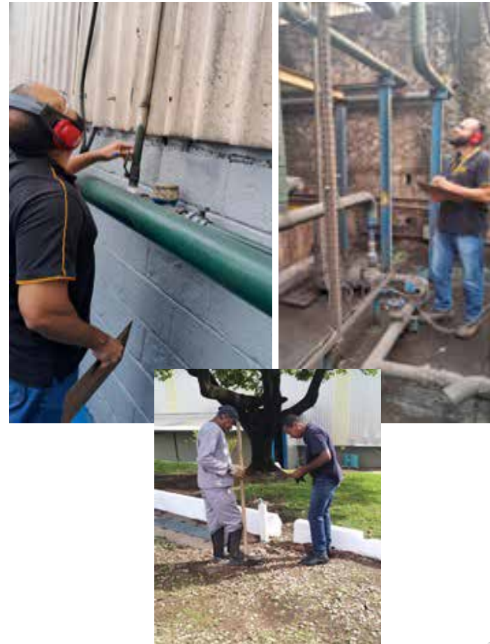
Associates inspected and fixed water pipes at our facilities in Brazil to stop leaks and conserve water.
