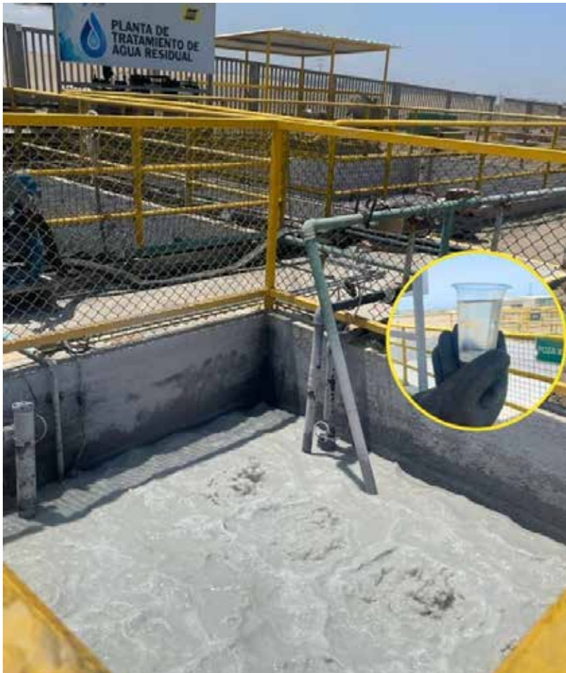
The treatment system at our facility in Peru removes contaminants from wastewater so the filtered water (inset) can be reused at our facility.
